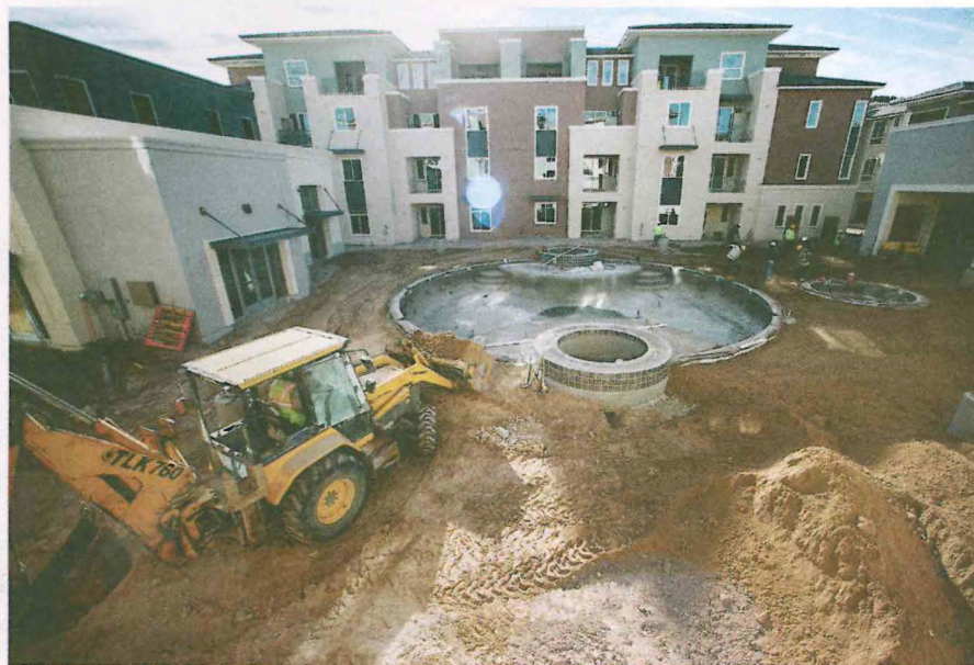
▶ A pool is under construction at Elysian at the District at Green Valley Ranch, an apartment complex at 2151 Village Walk Drive, Henderson. (MIKAYLA WHITMORE/STAFF)
